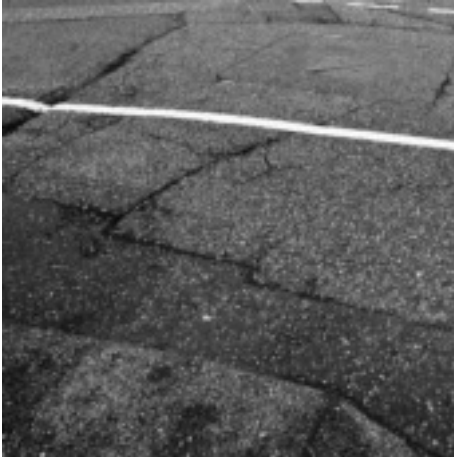
the High Street – Third World road surface
